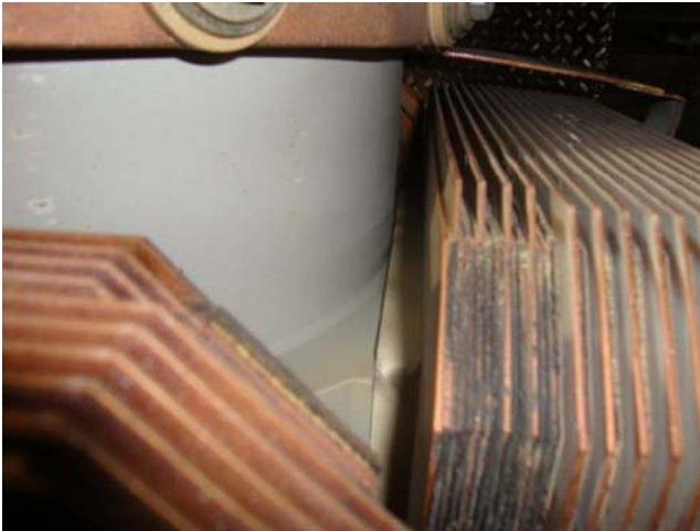
Figure 10.4 Contamination of a strip-on-edge field winding pole.
