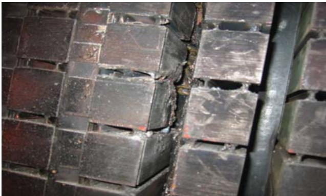
Figure 13.4 Damage to stator core from winding ground fault in slot.
