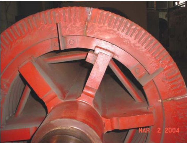
Figure 12.6 Cracks in shorting ring of high inertia drive motor due to low cycle fatigue.
