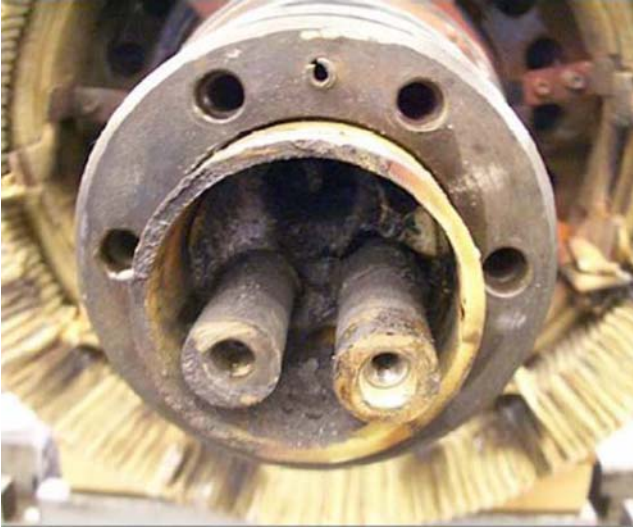
Figure 11.2 Rotor winding lead insulation failure from interphasal partial discharges.
