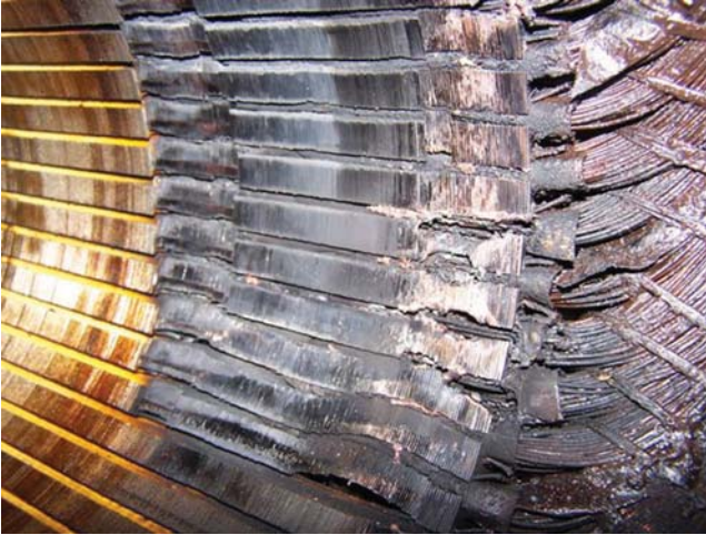
Figure 13.10 Stator rub on bore from bearing failure.
