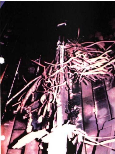
Figure 8.13 View of the stator bore (after rotor removal) of an 800 MVA turbogenerator that experienced a phase-to-phase fault in the stator slot. The white “spaghetti” are the copper conductors that came out of the stator slot under the tremendous magnetic forces that accompany a phase-to-phase fault.
