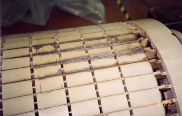
Figure 12.5 Rotor core burning resulting from broken bars.
