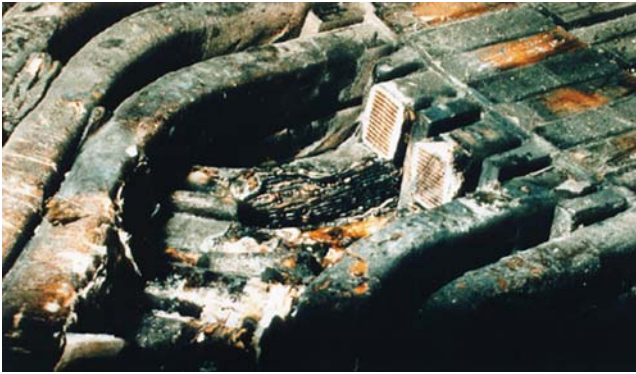
Figure 8.14 A turn-to-turn failure leading to a ground fault on a 6.6 kV, 8 MW motor. A bottom coil experienced the failure, and the top coils were cut away to expose the fault.
