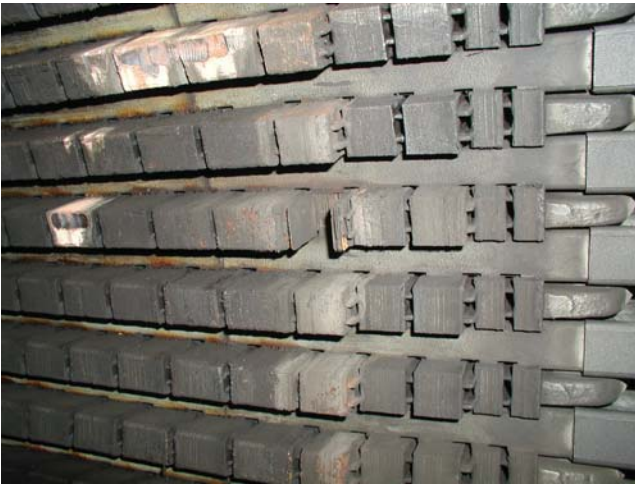
Figure 13.11 Core damage from a loose bolt.
