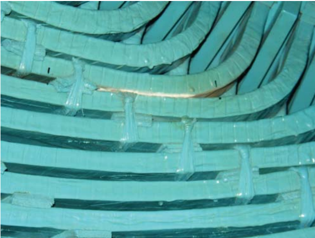
Figure 8.20 PD between adjacent coils in different phases results in white powder on the stator bar surfaces.
