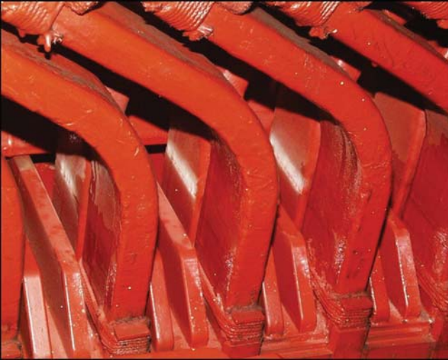
Figure 8.10 Photograph of the end winding area from a hydrogenerator. The white band around some of the coils just outside the slot indicates where the coating overlap area has degraded. Note that the entire stator has been painted with an abrasion resistant coating that makes repair of the overlap problem very difficult.
