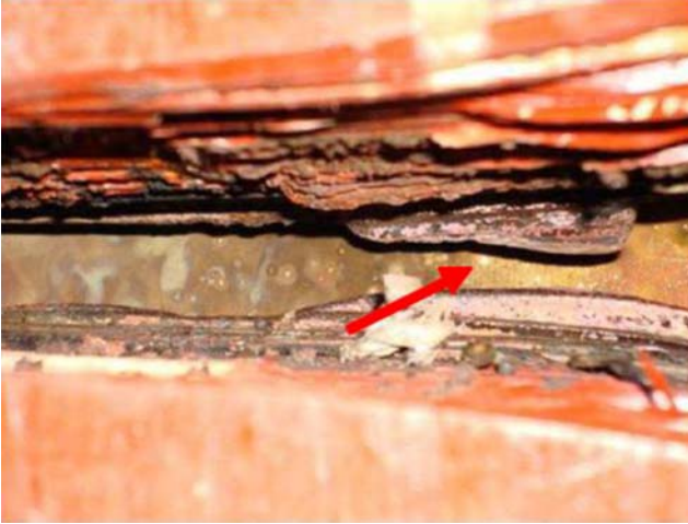
Figure 9.3 Failed pole jumper connection.
