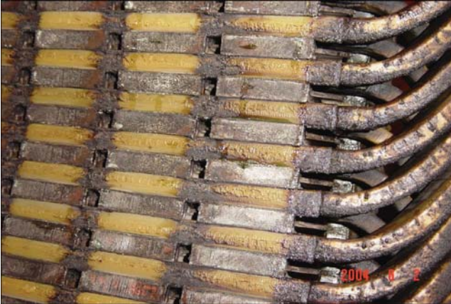
Figure 8.18 Photo of a stator winding degraded by acids in chimney flue gas. (See color plate section).
