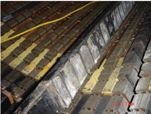
Figure 8.12 A stator bar being removed from an air-cooled turbine generator affected by VS.
