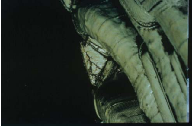
Figure 8.17 A photograph of a carbonized (black) track across a block between two coils in different phases in the end winding.
