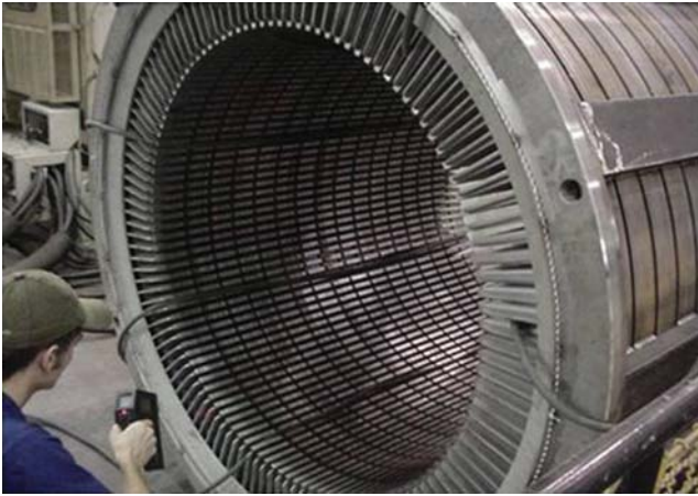
Figure 17.3 Excitation winding made from insulated cable wound through a stator core.
