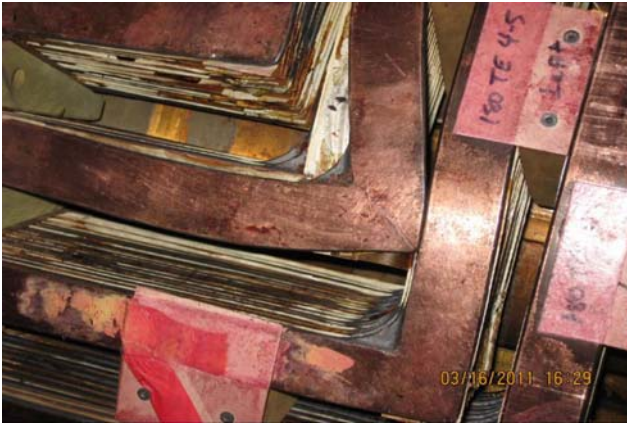
Figure 9.2 End winding copper distortion from thermal cycling.
