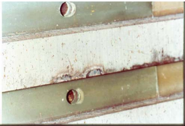
Figure 13.3 Localized core overheating from core insulation thermal aging.
