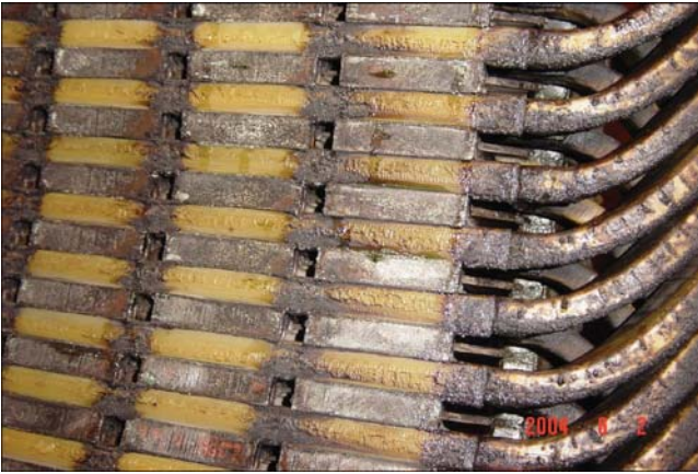
Figure 8.18 Photo of a stator winding degraded by acids in chimney flue gas.
