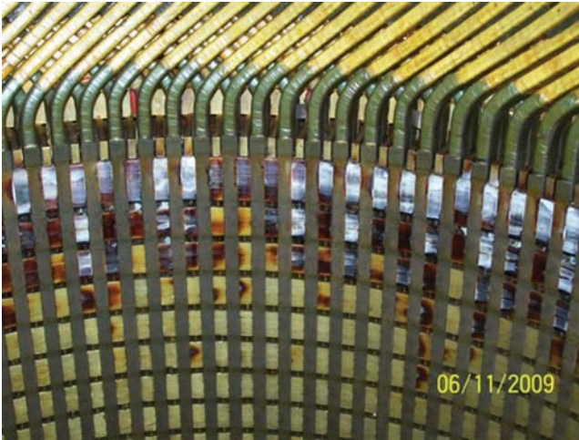
Figure 13.2 Stator core burning that resulted from excessive oven temperatures during stator winding burnout prior to rewind.
