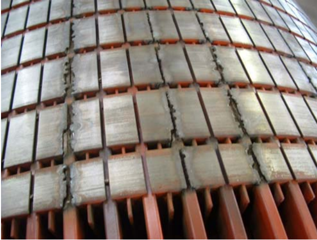
Figure 12.8 Core bridge burning due to loose bars in slots (Source: Courtesy of EASA).
