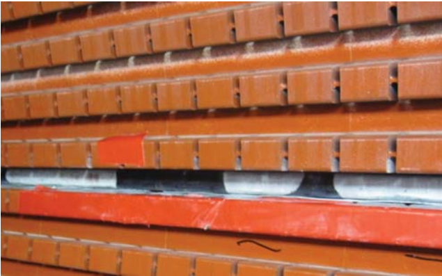
Figure 8.8 Photograph of a stator slot taken from the axis of an air-cooled machine. The stator wedges have been removed in one slot, exposing the top of a coil. The semiconductive coating on the coil connected to the phase terminal has disappeared (turned white). (See color plate section).
