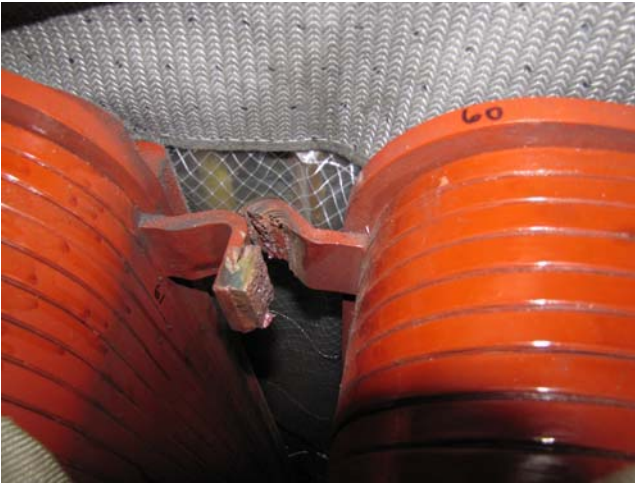
Figure 10.3 Failure of inter-pole connection from thermal cycling.
