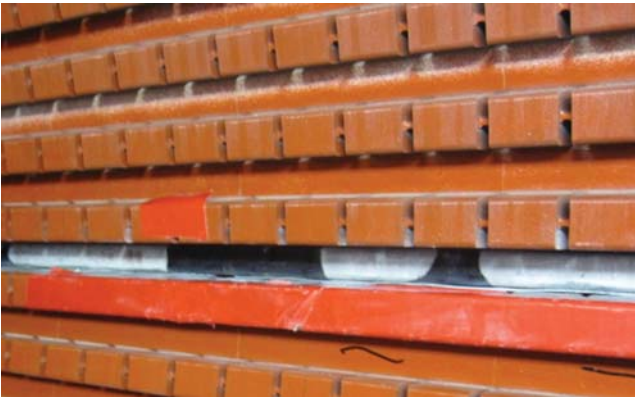
Figure 8.8 Photograph of a stator slot taken from the axis of an air-cooled machine. The stator wedges have been removed in one slot, exposing the top of a coil. The semiconductive coating on the coil connected to the phase terminal has disappeared (turned white).
