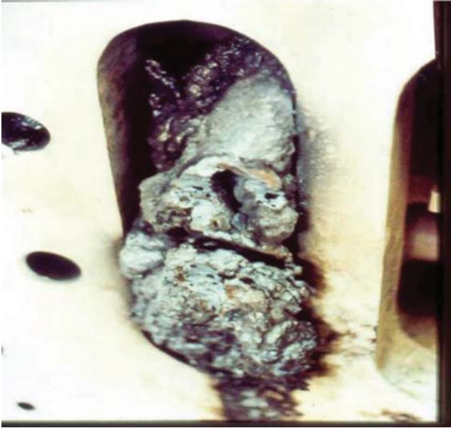
Figure 13.8 Massive core melting with molten steel coming out of the axial vent ducts in a large turbo generator.
